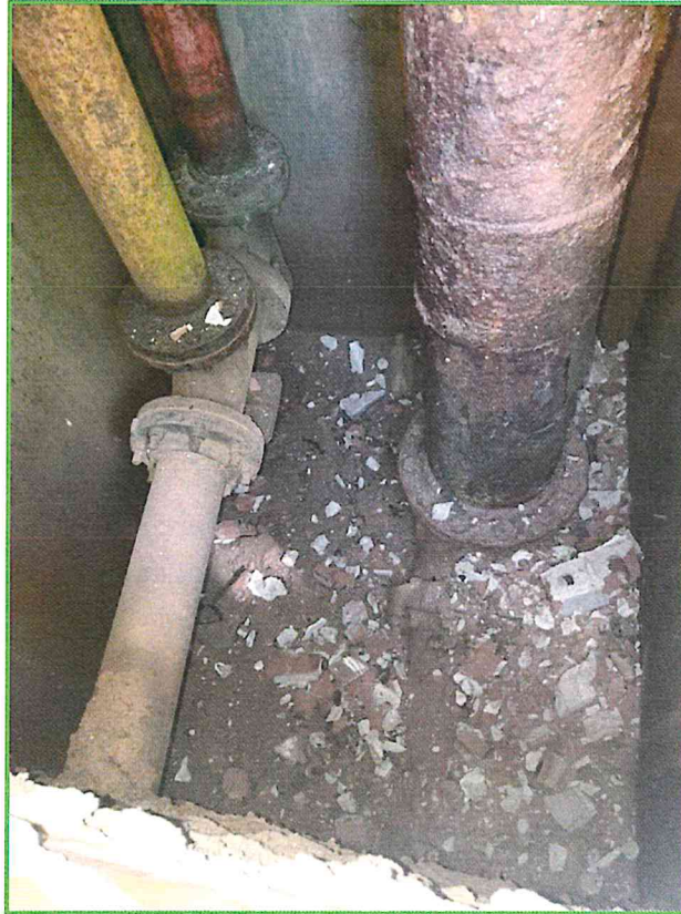
Figure 1 - Memory Lane Water Vault
